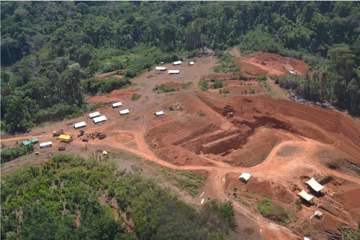
Figure 25: Sapolite mining at the Randy pit within the IAMGOLD drilling grid on October 6, 2022
